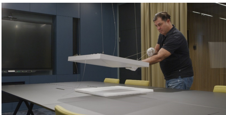
The Sennheiser ceiling microphone was supplied, installed and set up by Supravisio AG
